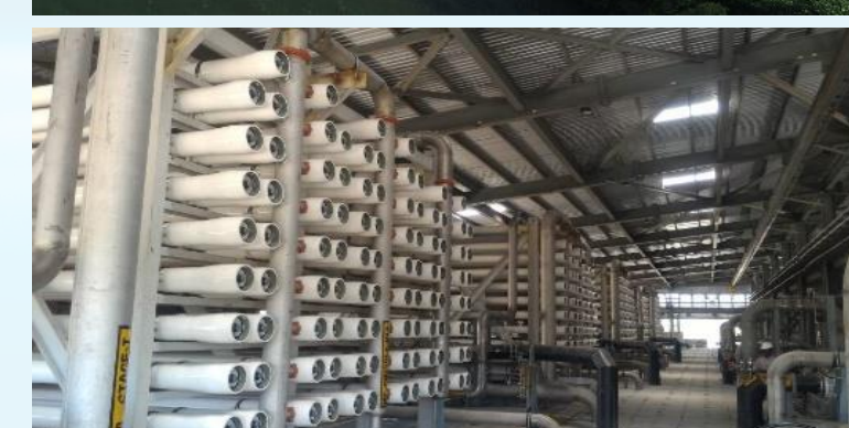
50 MLD BWRO (Desalination), for Reliance Industries, Dahej, India Turnkey project executed in record 8 months 24 days
