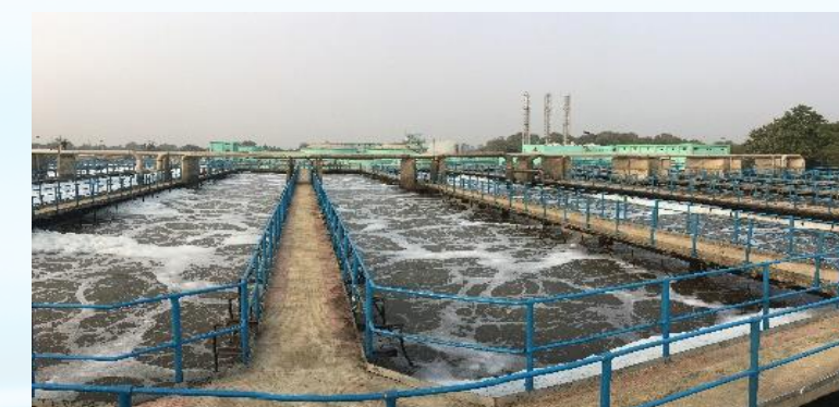
140 MLD Sewage Treatment Plant, Dinapur, Varanasi, India First and largest STP to be inaugurated under 'Clean Ganga' mission
