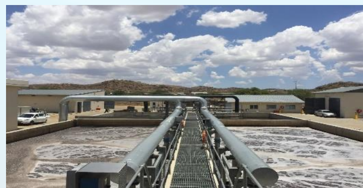
5 MLD Industrial Water Reclamation Plant, Ujams, Windhoek, Namibia First plant of its kind in Namibia, treating effluents from five different production facilities 21 MLD New Goreangab Water Treatment Plant, Windhoek, Namibia First worldwide direct potable water reuse plant.
