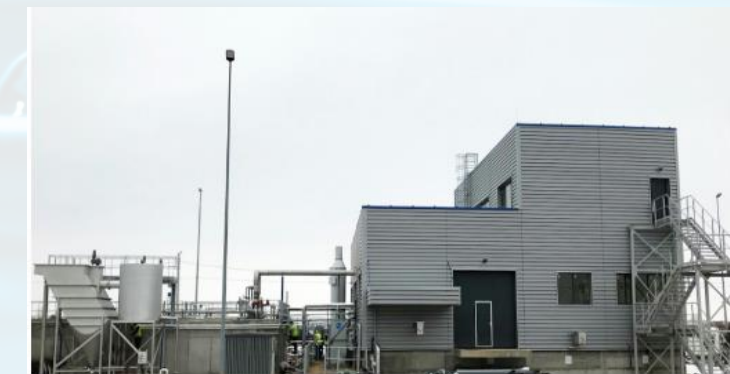
Industrial Effluent Treatment Plant for Phillip Morris, Otopeni, Bucharest, Romania Treatment of effluents from tobacco production
