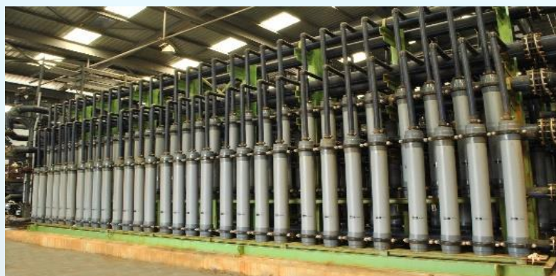
110 MLD SWRO (Desalination) Plant, Nemmeli, Chennai, India India's largest operational desalination plant till date
