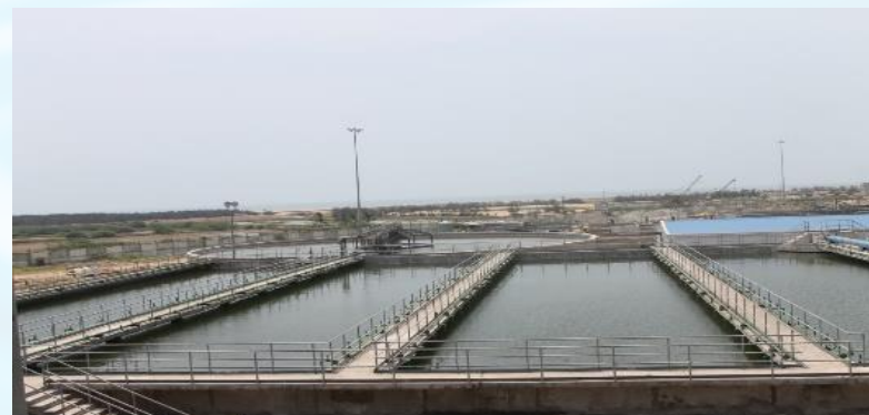
54 MLD Effluent Treatment and recycling plant, for Indian Oil Corporation Limited, Paradip, Odisha, India India's largest industrial water recycling plant
