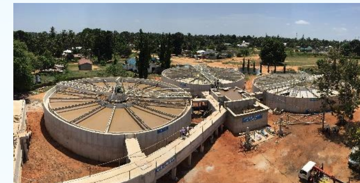
130 MLD Drinking Water Treatment Plant, Tanzania First water project in Africa to be commissioned under EXIM India funding
